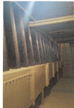
Refurbished Air inlet filter house. (interior)
