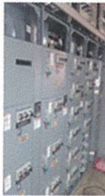
New 480VAC MCC panel Switch Gear
