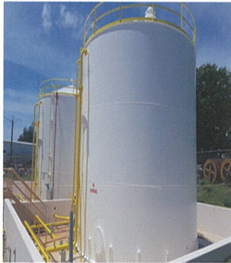
Fuel Tanks Integrity testing complete and re-filled with ULSD fuel
