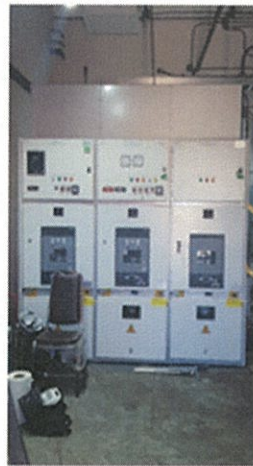
New 13.8KV Metal Clad Panels
