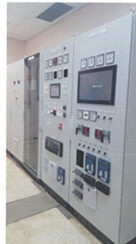
New Turbine Control System
