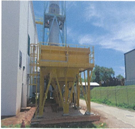
New Cooling Tower Structure Construction of 8" berm wall ongoing as required by SPCC
