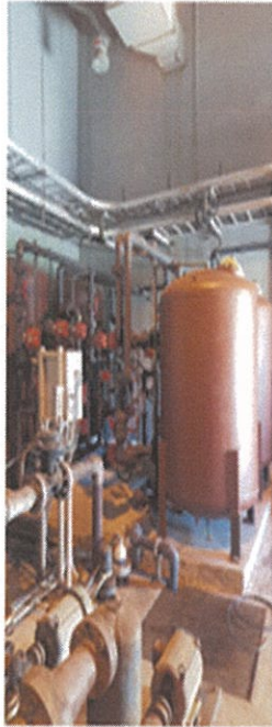
New Water Treatment System Multimedia filters & Carbon Filters
