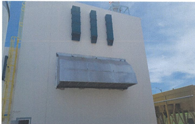
New Air Inlet Filter house Exterior hood.
