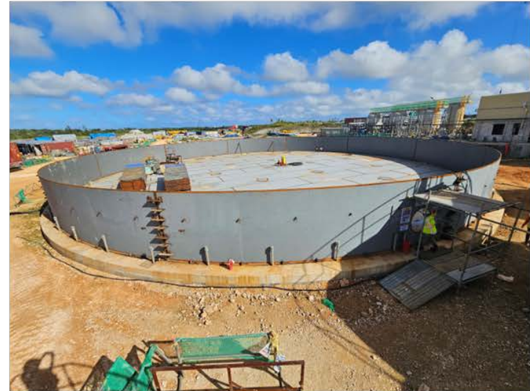
Treated Water Storage Tank B – Restoration of tank walls is in progress.
