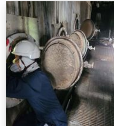
Plant personnel assessing for safe entry into boiler to make necessary repairs to 48-year-old Cabras Unit 2 baseload plant.
