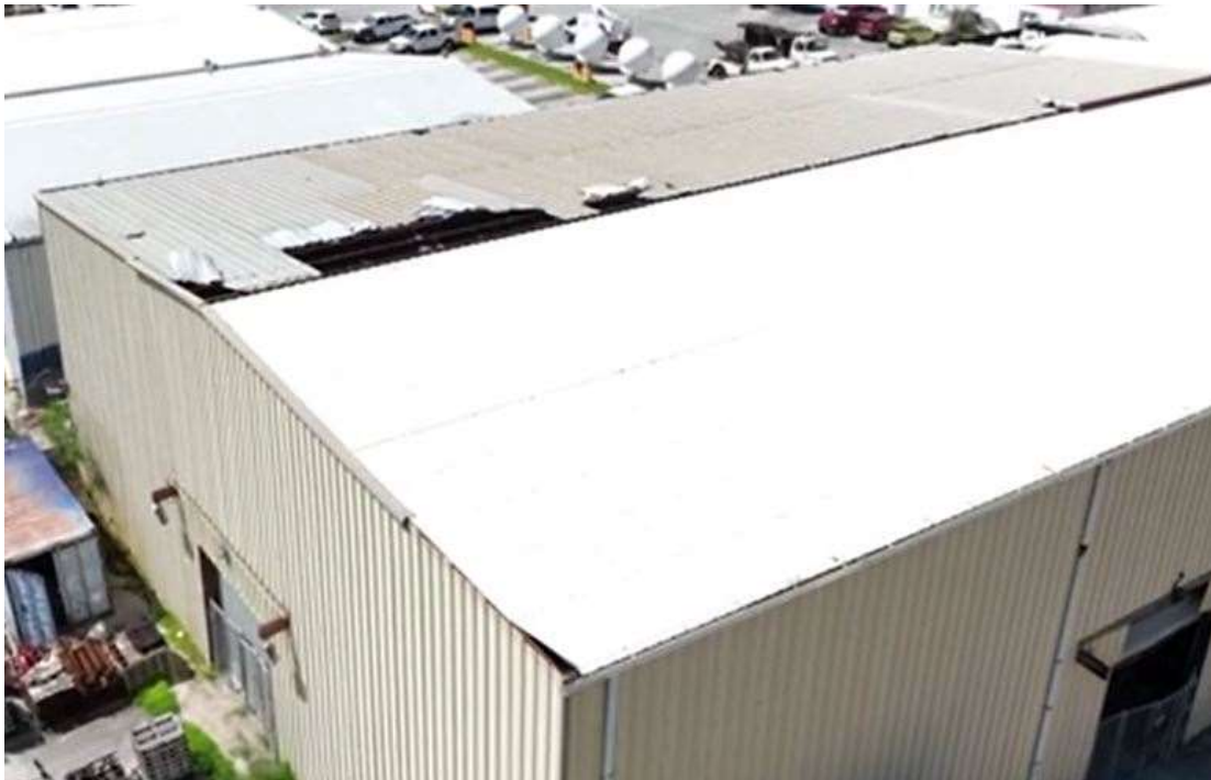
ITEM 7 & 7A – DAMAGED ROOFING NEAR THE RIDGE OF THE WAREHOUSE
