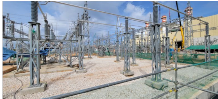
Switchyard – Gravel is being placed in the east side of the AIS yard
