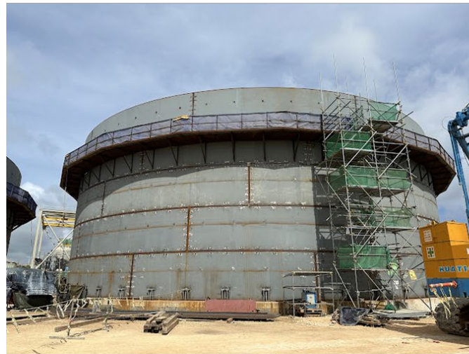
Treated Water Storage Tank B – 5 Courses of Steel Walls are in place
