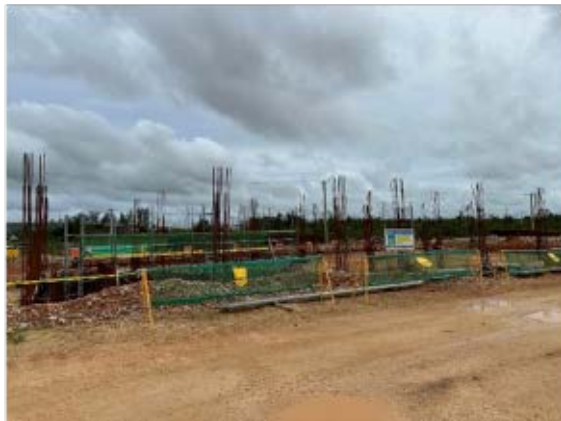
Admin Building – Rebar bent slightly.
