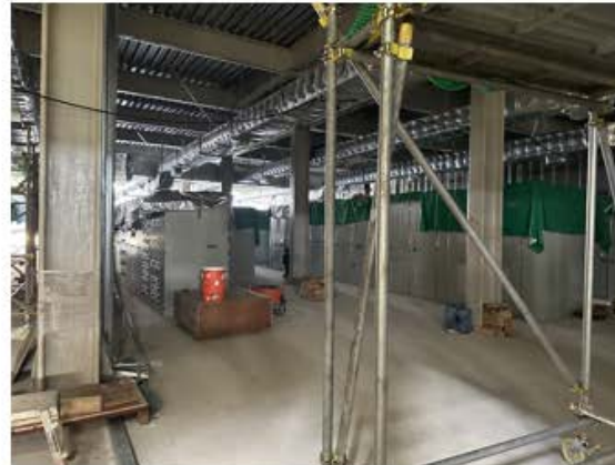
2 nd floor- Switchgear damage assessment ongoing
