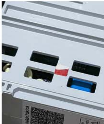
Sticker indicating water inside medium voltage protective relays
