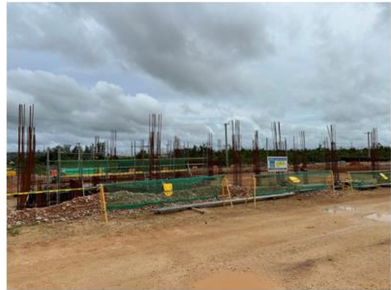
Admin Building – Rebar bent slightly.
