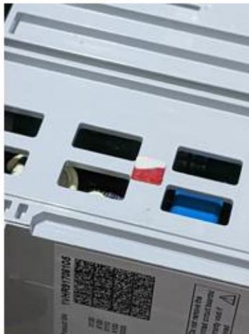
Sticker indicating water inside medium voltage protective relays
