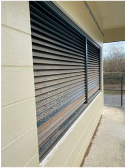
Clean Exterior Louvers
