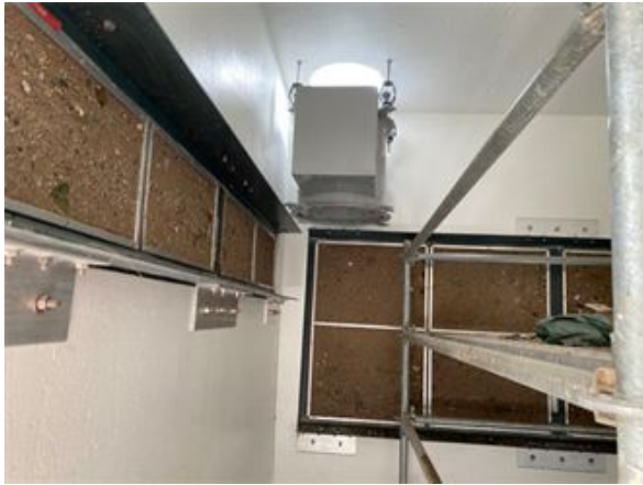
Clean Louver Screens
