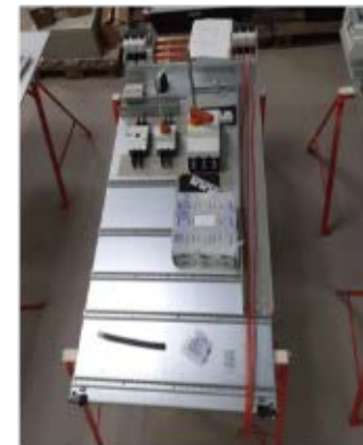
Fuel Oil Treatment System – Switch gear production in progress
