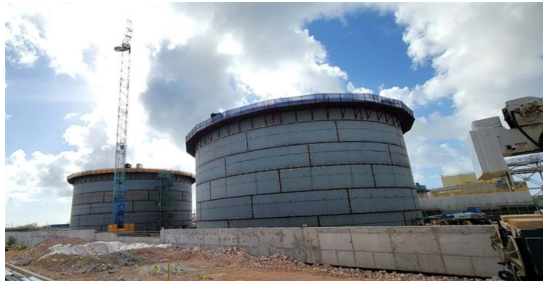
ULSD Storage Tanks – Both Tanks have all 6 courses of steel walls in place
