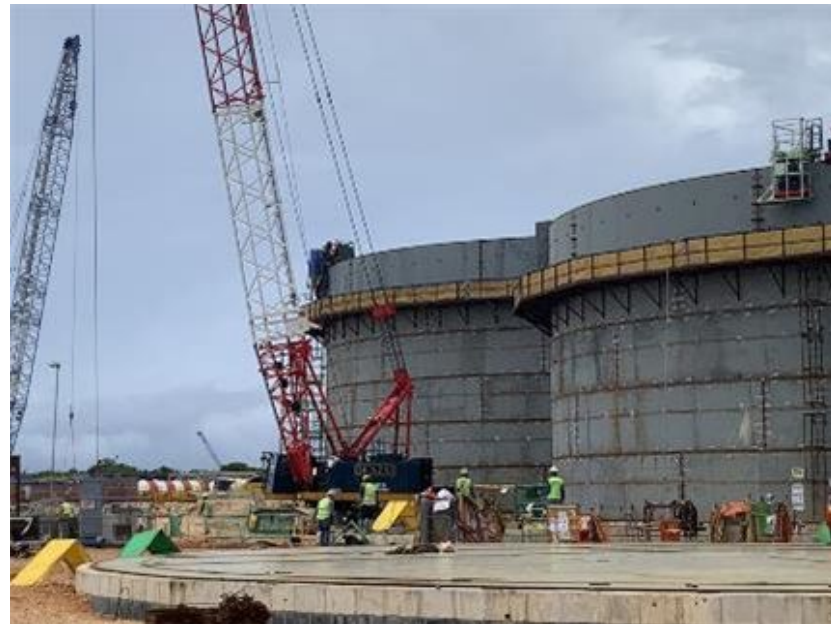
Treated Water Storage Tank 2 – Welding in progress for the 6 th (of 8) row of steel plates
