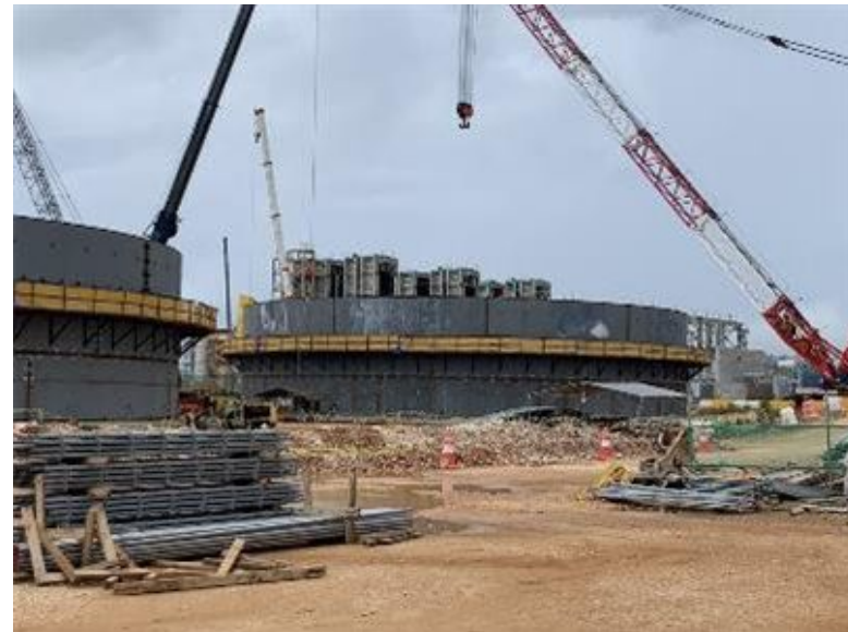
ULSD Storage Tank B— 3 rd Row of Steel Plates Currently Being Welded
