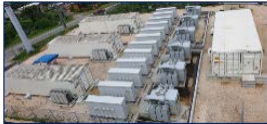
Hagåtña 24 MW Energy Storage Batteries
