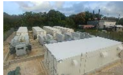
Talofofu BESS 16 MW Frequency Regulation
