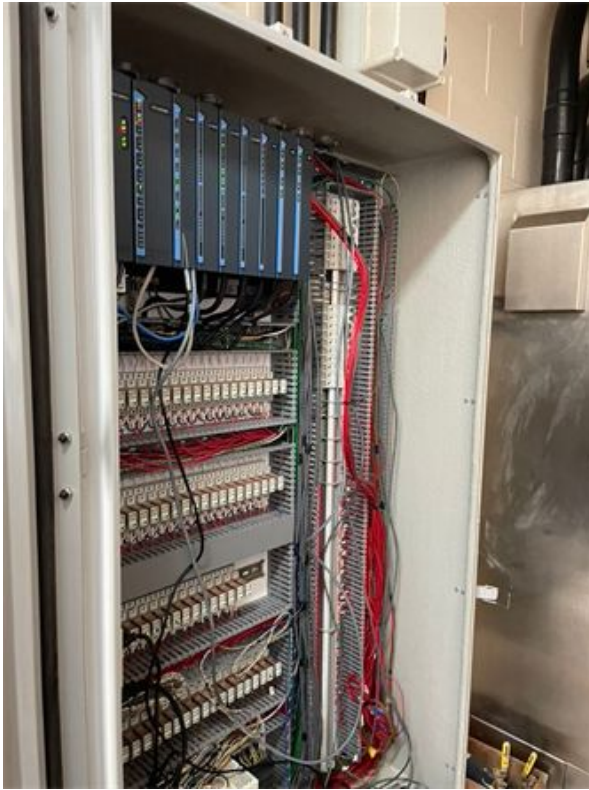
Chemical Room PLC
