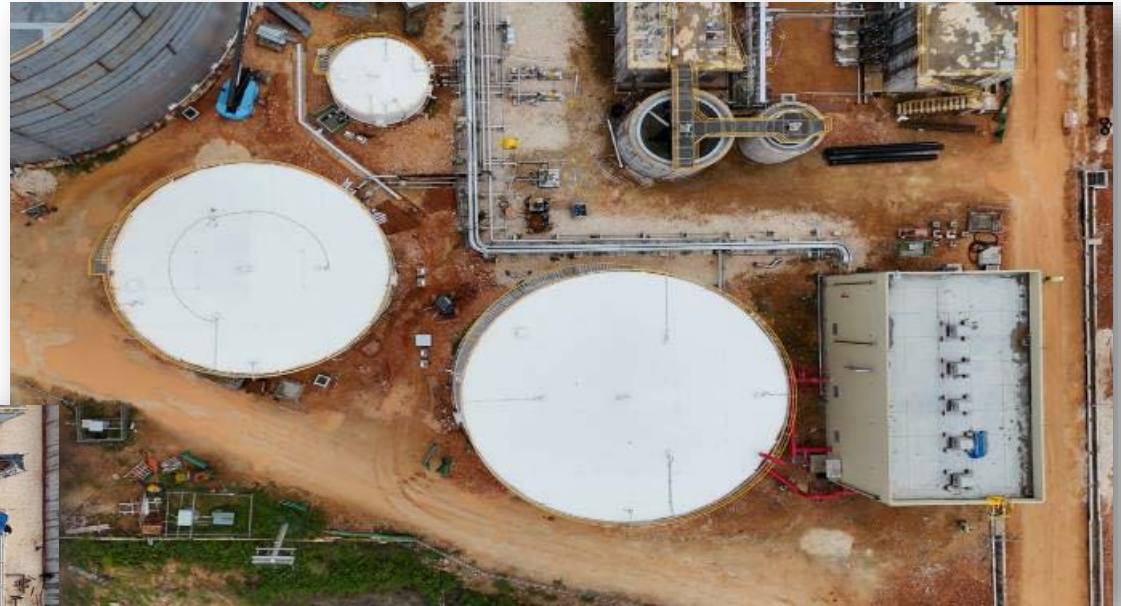
Fire Fighting Tank: Fire tank has been completed and filled with water.
