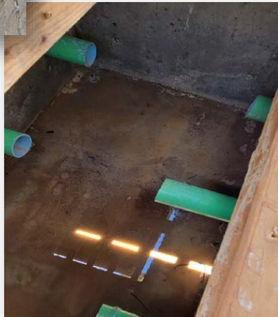
Inside of lifting station
